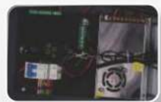
Pre Programmed Control Unit
